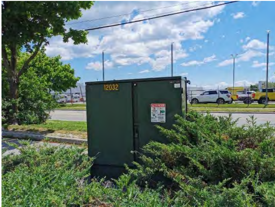
Photo 7: Transformer at 217 Cross Avenue, facing south.
