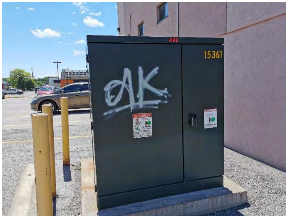
Photo 8: Transformer at 581 Argus Road, facing west.
